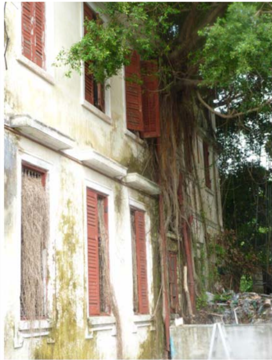
Detail View of Damage from Tree Growing on Building
